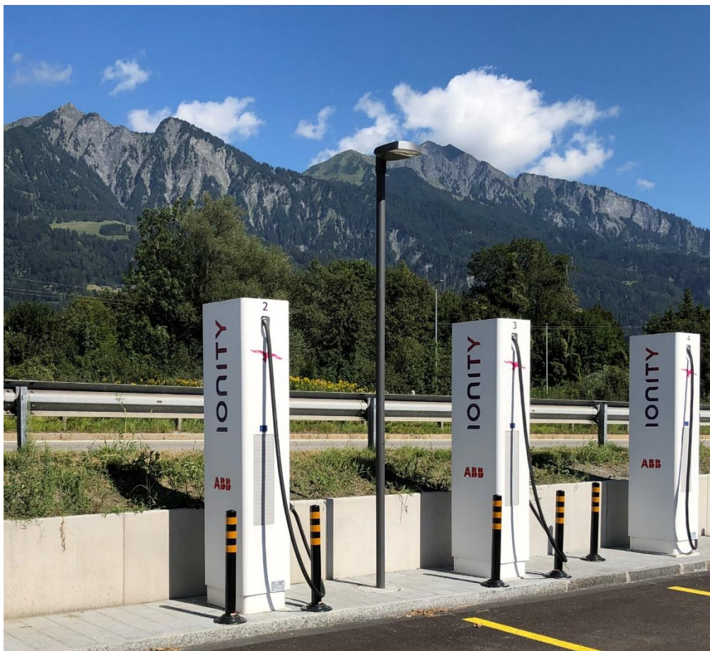
EV Charging Stations, Bad Ragaz, Switzerland
